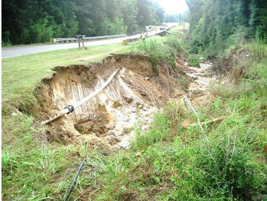
Figure 6. Bed incision in the main channel has triggered a valley trench gully up the side of this road, Alabama. Note exposed utility pipeline.
