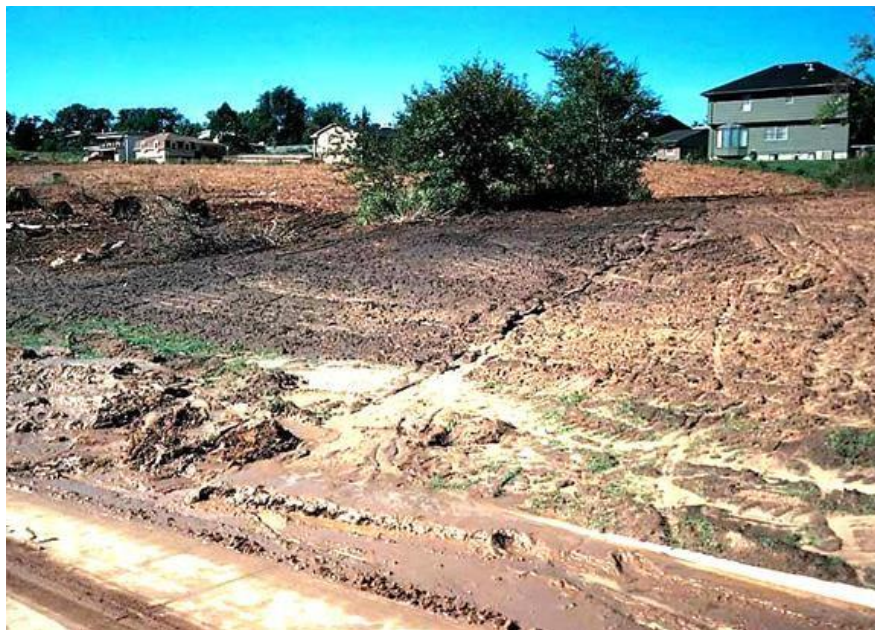
Figure 12. Severe sheet and rill and gully erosion resulting from recent construction.
